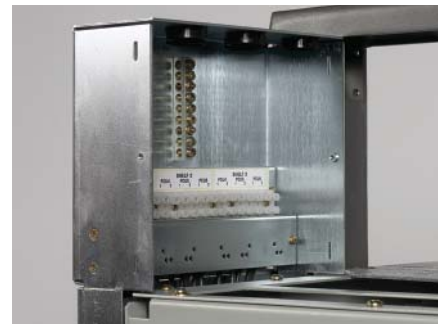
Top AC Wireway Input (cover removed)
