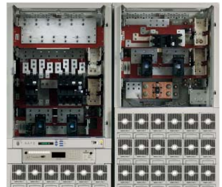
Modular Distribution Cabinets
