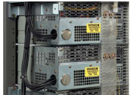
Bottom AC Wireway Input (cover removed)
