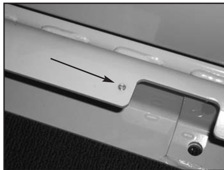
Figure 2: Adequate Paint Penetration
